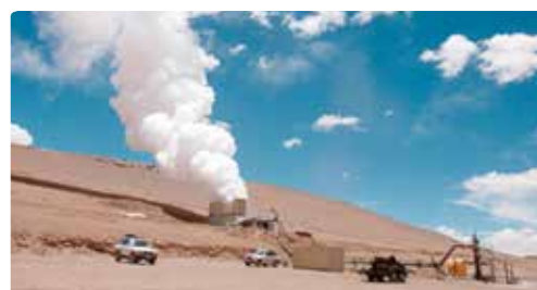
A fumarolic gas test being carried out for the Laguna Colorada Geothermal Power Plant Construction Project (Bolivia)
